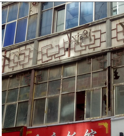
舟曲县南门商场楼窗户现状
